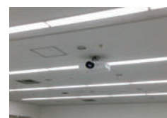
Built-in projector on ceiling
